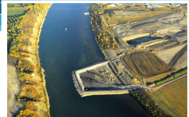
The southside river berm allows crews to build the first half of the North Saskatchewan twin bridges.
